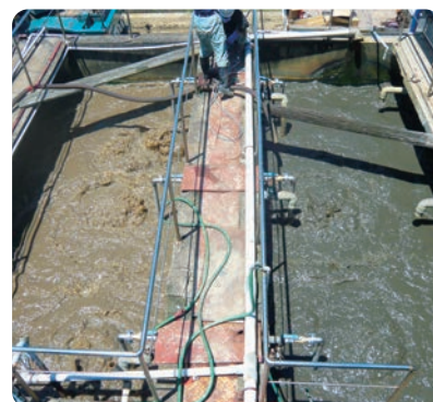
Aeration tank running condition
