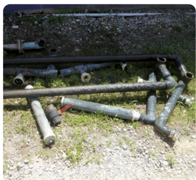
Existing diffuser deteriorated and damaged due to clogging
